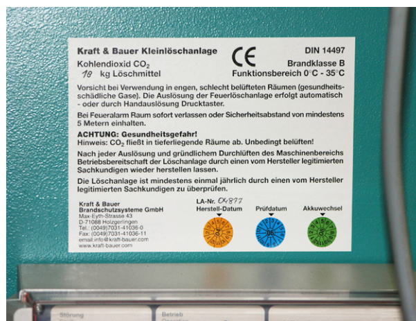
Example: Inspection stickers Kraft & Bauer
